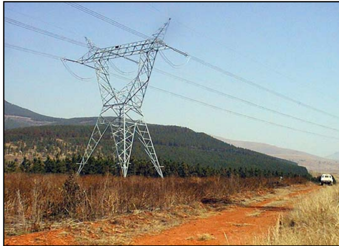
Figure 3: Self-Supporting Strain Tower
